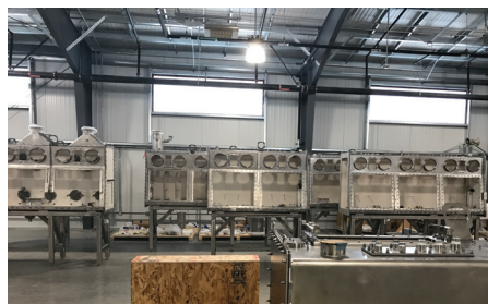
The glovebox trains awaiting installation into RLUOB laboratory space.
