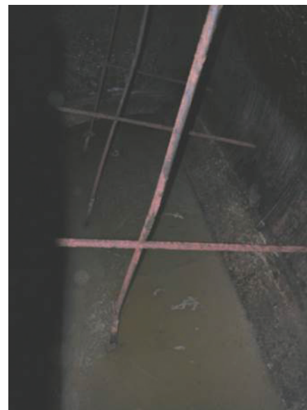
The inside of one of the General's Tanks before sampling. Most of the liquid was removed when the tanks were partially excavated in 1974, leaving only this thin layer over the sludge at the bottom of the tank. Some of the sludge is barely visible at the lower left, next to the pink rod.
