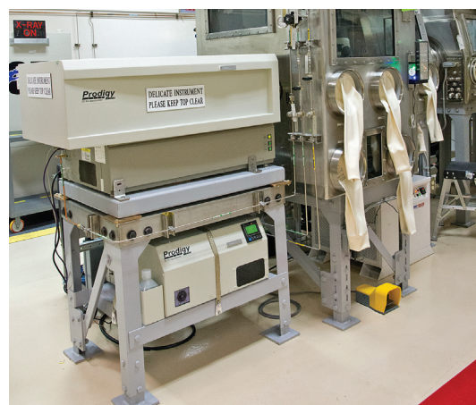
The new Prodigy DC arc instrument installed in PF-4 is just over a meter long. The sample chamber is radiologically contained in the glovebox, while the optics and computer controls are on the stand outside the glovebox.
